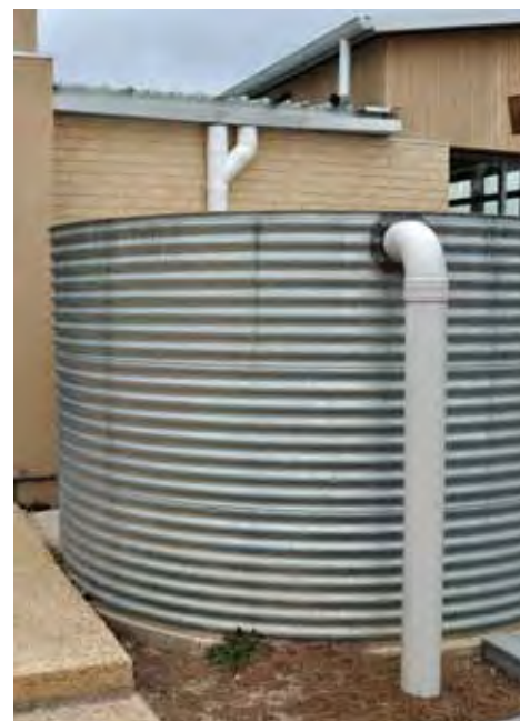
Rainwater collection system
