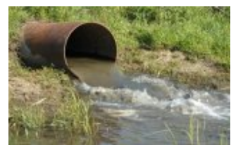
Discharge from NPDES outfall
